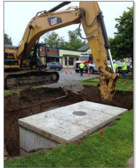
The Village installs one of the stormwater cisterns underground adjacent to the parking lot in front of Dave's Diner on Albany Street.
